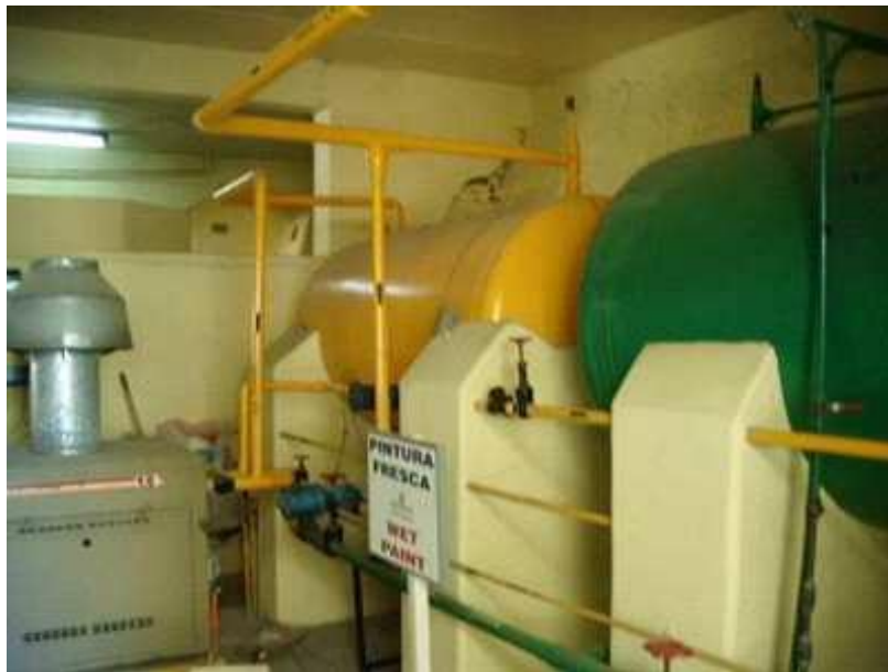
The Hot and Cold Water Tank System Replacement has been included in the Study under the Category "Building Interior" along with remodel of the Office Areas and Storage.
