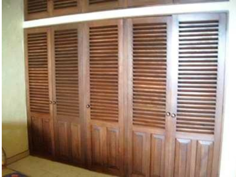
The Closet Doors are made of wood and are in overall very good condition, especially considering their age. Replacement of these doors has not been included in the Study.
